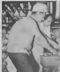
Janita Warlaman, supervisor Mech.-M&C, and Danilo Danieli, Nuovo Pignoni, help install high-speed centrifugal recycle compressor for hydrogen gas.
